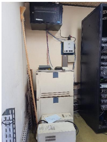
FIG 20 - Rack F Sala do DG
