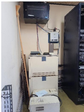
FIG 20 - Rack F Sala do DG
